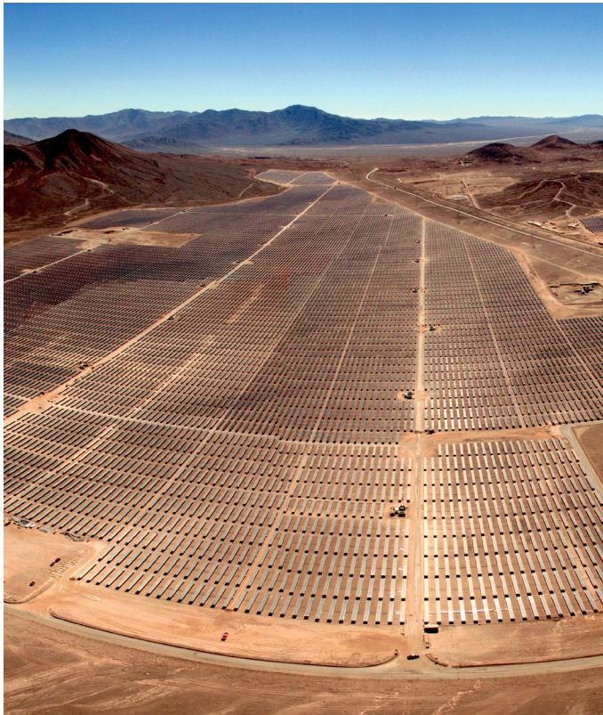
Utility-scale solar photovoltaics in Chile's Atacama Desert.
